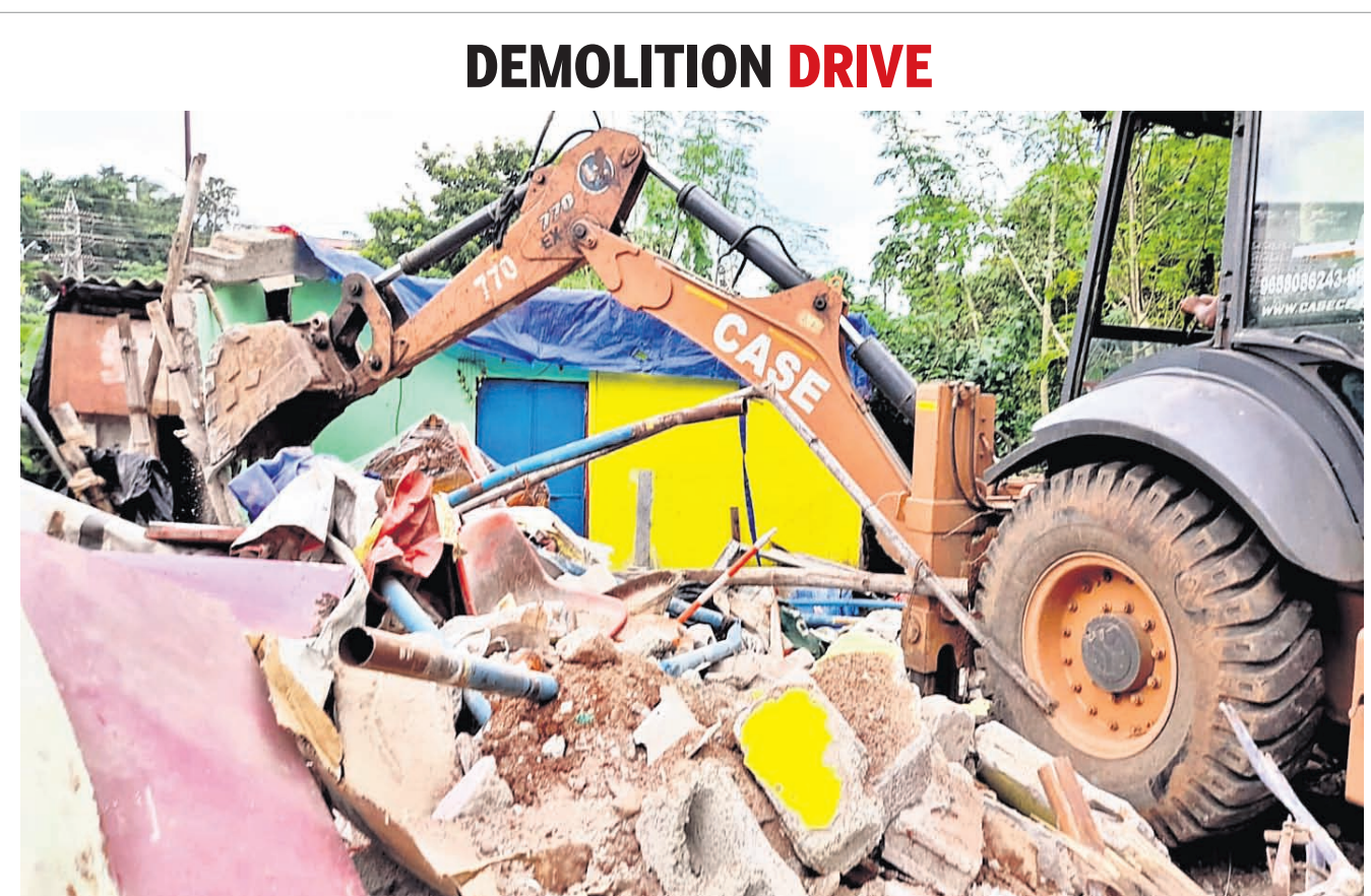
An excavator demolishing an illegally constructed house belonging to drug peddler and murder accused Ranju Naik in Unit-VIII area of Bhubaneswar, Saturday
