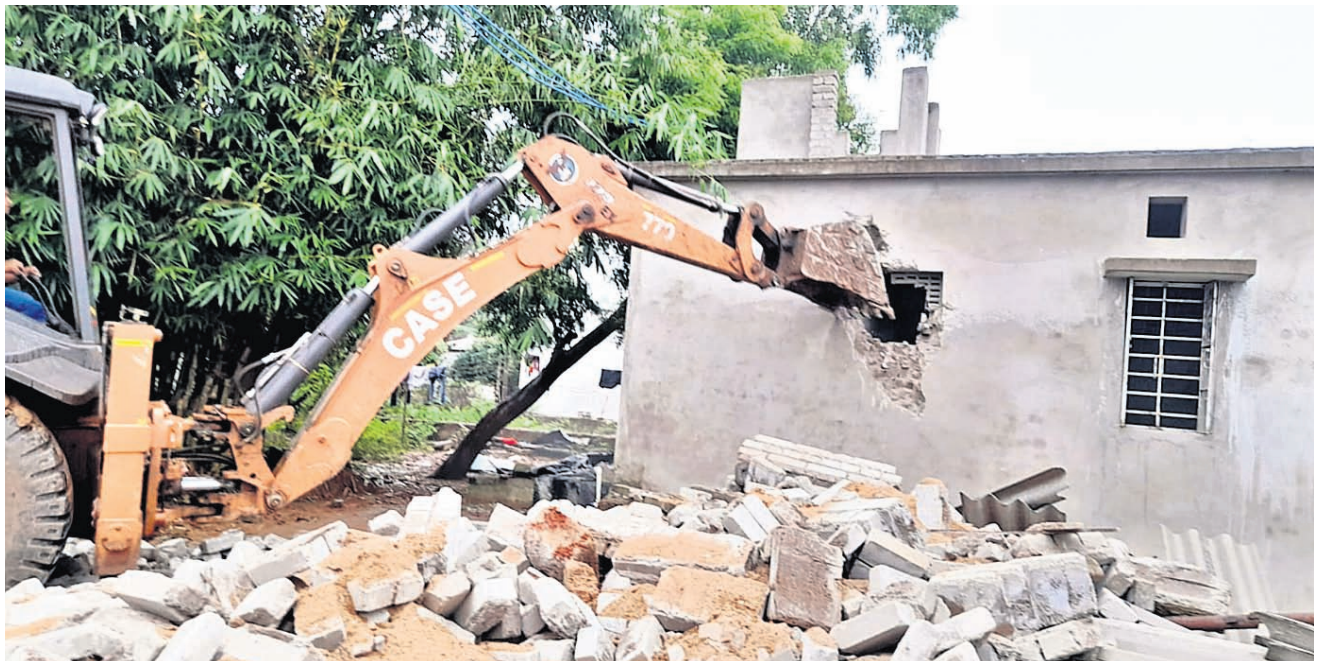
An excavator deployed by BDA razing down an illegally constructed house at Shyampur under Khandagiri police station in Bhubaneswar, Monday
