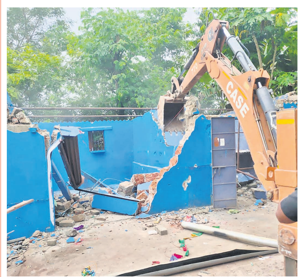
DEMOLITION DRIVE: An excavator engaged by BDA demolished illegal structures near Kuakhai bridge in Bhubaneswar, Friday
