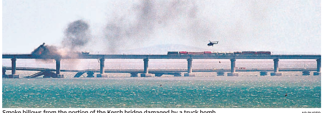
Smoke billows from the portion of the Kerch bridge damaged by a truck bomb
