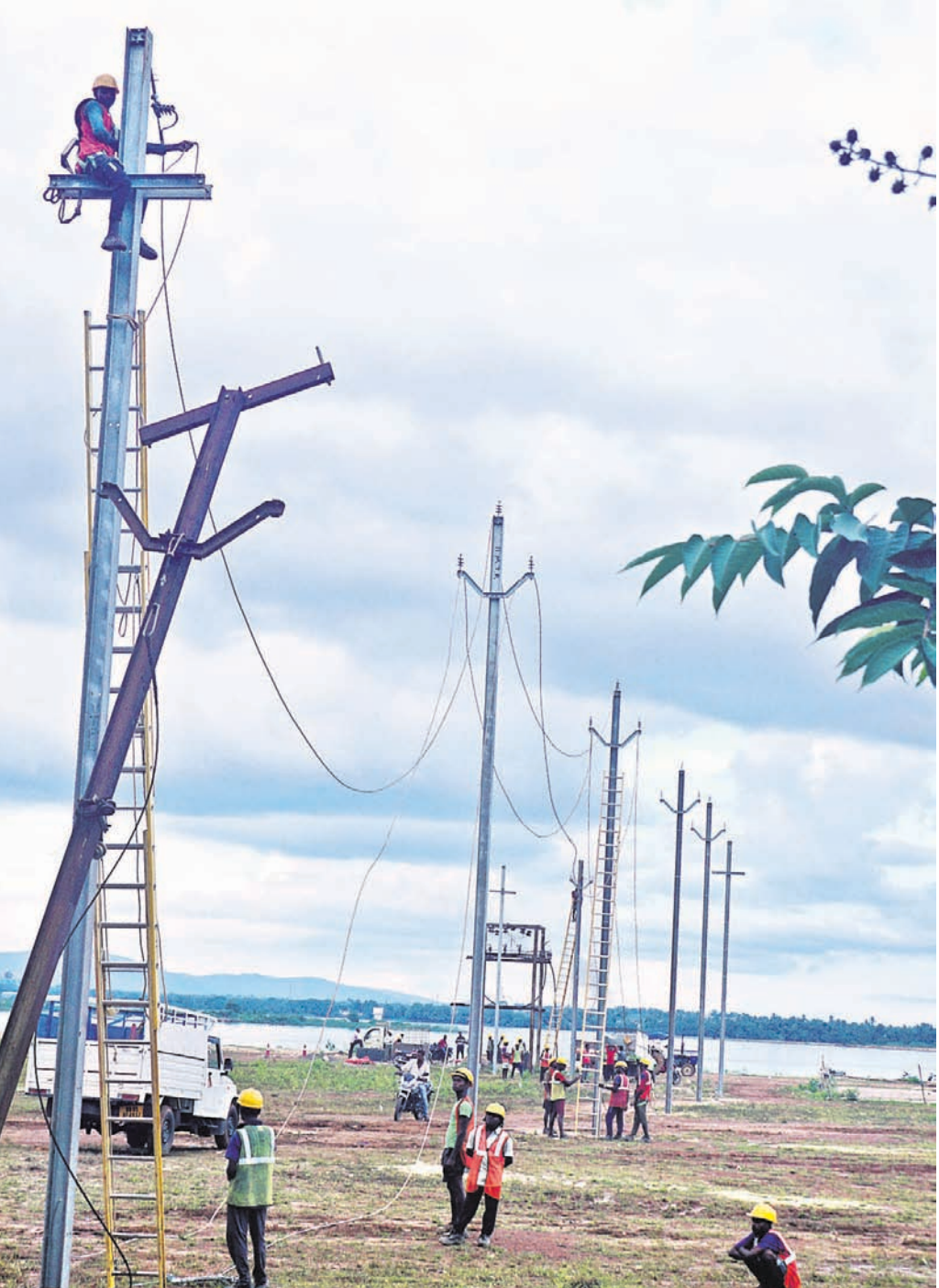
BALIYATRA PREP: Electricity connection to Baliyatra Lower Ground in progress in Cuttack, Saturday, as the Silver city is bracing for a curbs-free maritime fair after two years of Covid-19 pandemic
