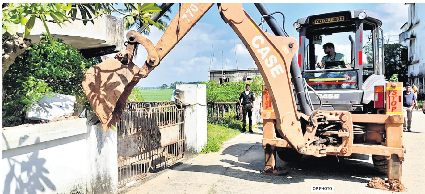
OP PHOTO RAZING DOWN: An excavator deployed by BMC flattening an illegally constructed house at Balakati Jhantisan area on the outskirts of Bhubaneswar, Thursday
