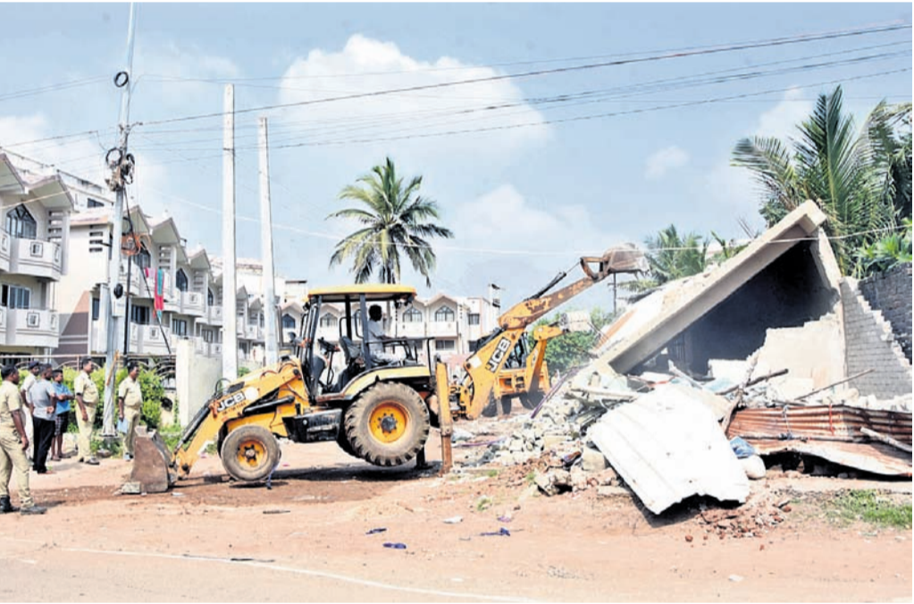
DEMOLITION DRIVE: An excavator engaged by the civic body pulls down an illegal structure in Puri, Wednesday OP PHOTO
