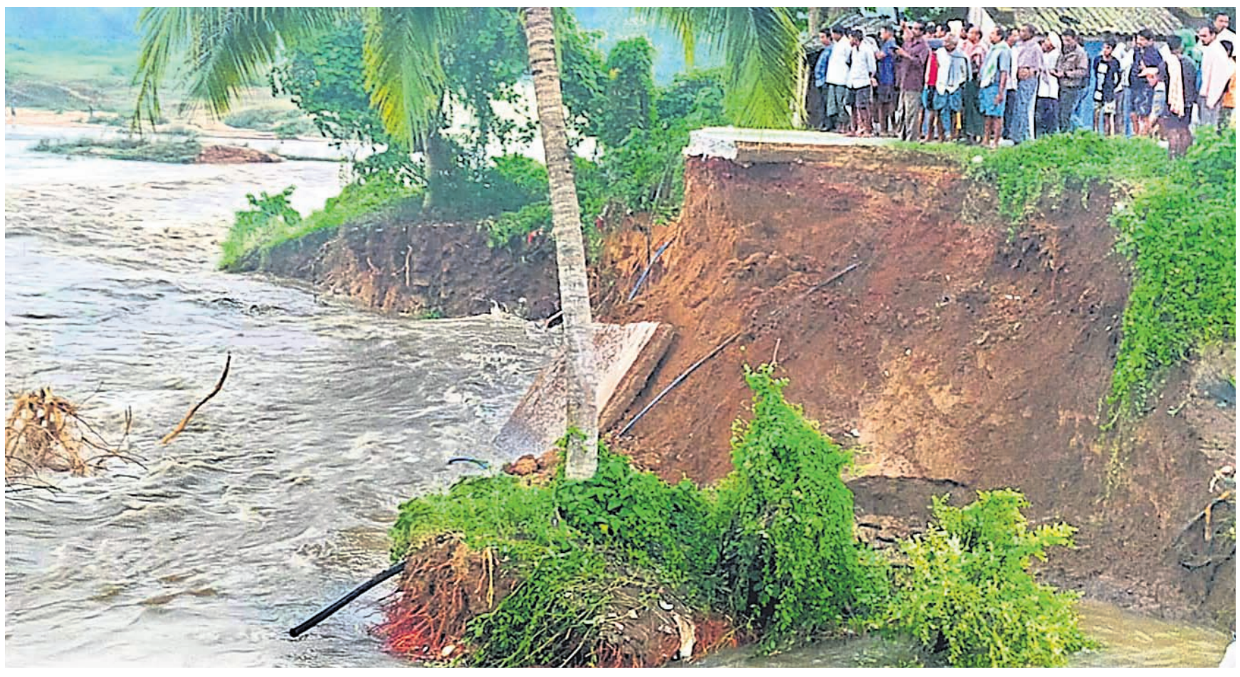
EMBANKMENT BREACH: People look at a 100-ft breach on Pattamundai canal embankment that washed away a two-storey building housing six shops at Trivenishwar market under Mahanga block in Cuttack district, Saturday (REPORT P7)
