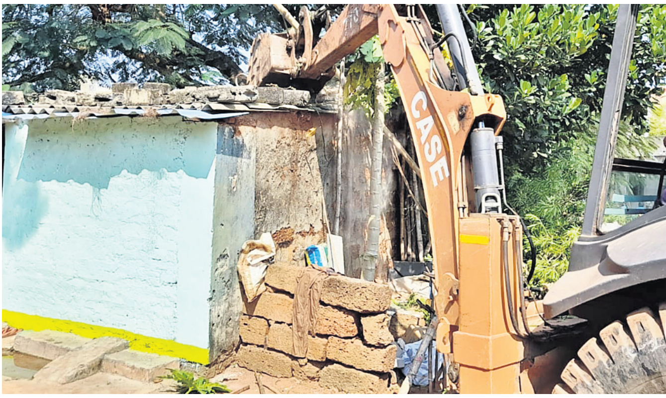
DEMOLITION DRIVE: An excavator deployed by the BMC pulls down an illegally-built house in the Dumduma area of Bhubaneswar, Tuesday OP PHOTO
