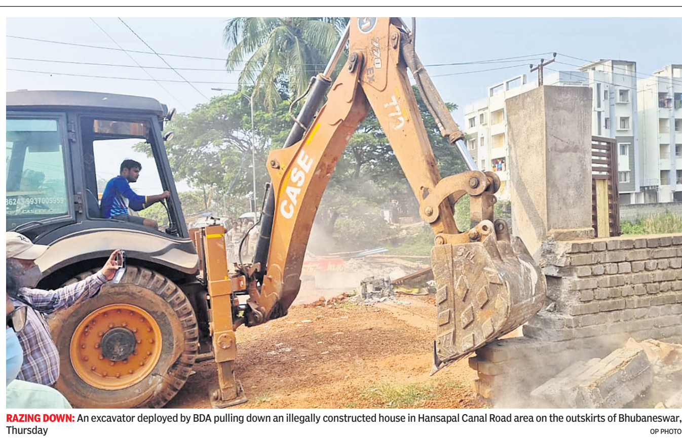
RAZING DOWN: An excavator deployed by BDA pulling down an illegally constructed house in Hansapal Canal Road area on the outskirts of Bhubaneswar, Thursday
