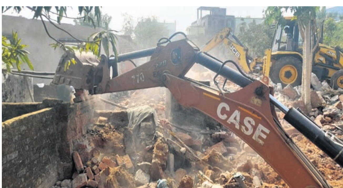
DEMOLITION DRIVE: An excavator deployed by BDA pulling down an illegally built house at Nicco Park road in Bhubaneswar, Monday
