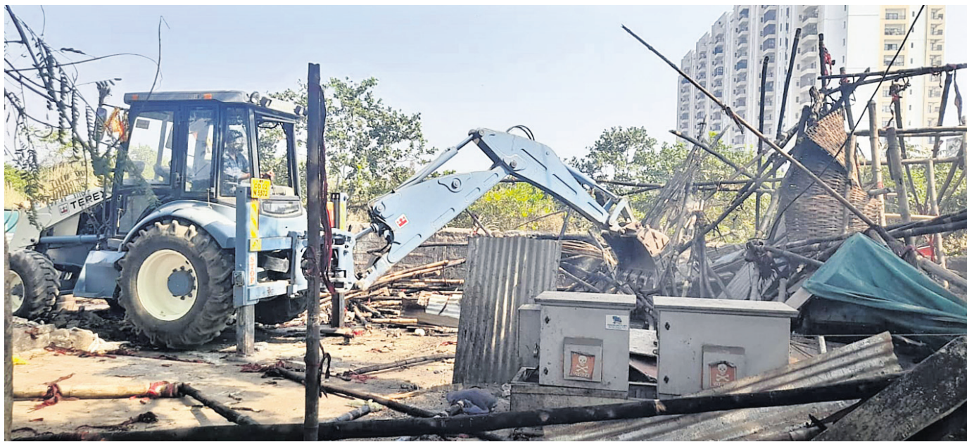
ANTI-ENCROACHMENT DRIVE: An excavator razing down illegal shops located along Patia Square to KIIT road in Bhubaneswar, Monday
