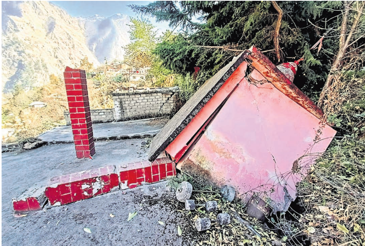
A temple collapses after the gradual 'sinking' of Joshimath in Chamoli district of Uttarakhand, Sunday
