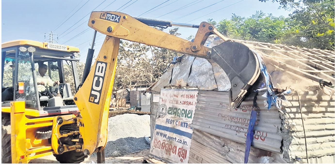
RAZING DOWN: An excavator deployed by BDA demolishing an illegally built structure at Aiginia in Bhubaneswar, Monday
