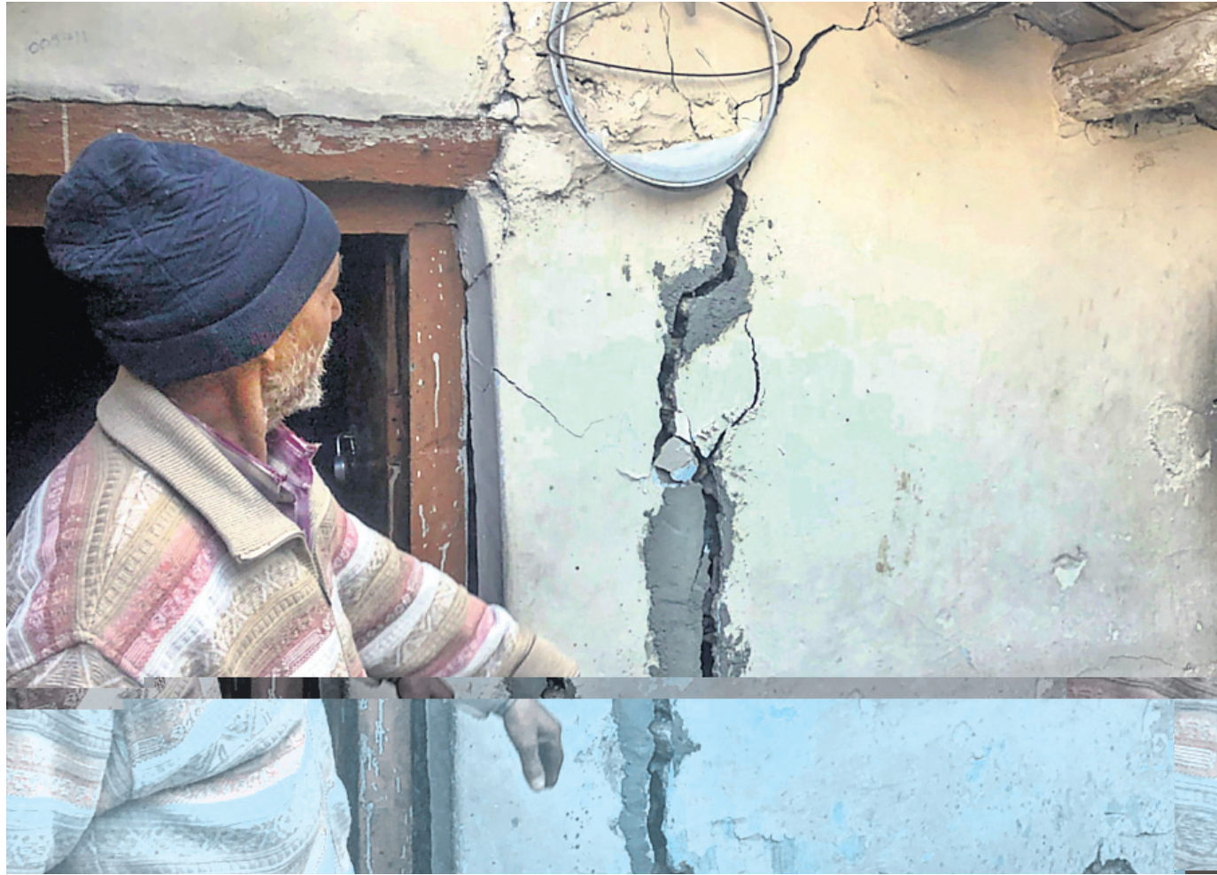
A man shows the cracks that appeared in his house at Joshimath in Chamoli district in Uttarakhand.
