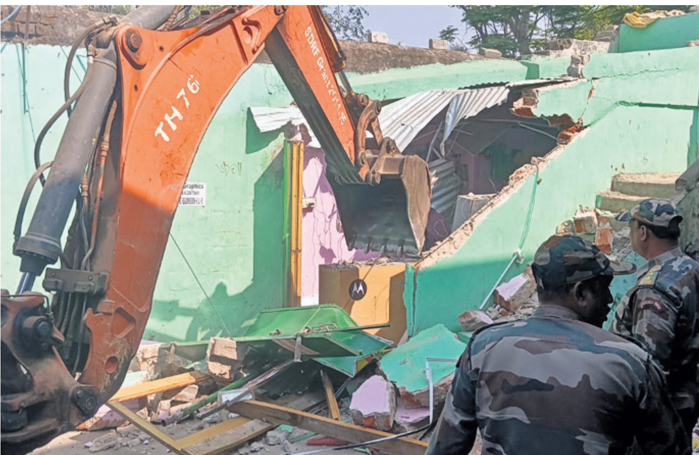
RAZING DOWN: An excavator engaged by CMC demolishing illegally constructed shops at OMP Market Complex in Cuttack, Tuesday
