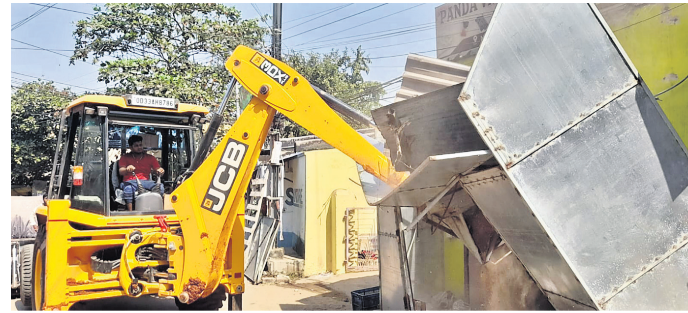
RAZING DOWN: An excavator engaged by BDA pulling down an illegally constructed house at Nayapalli in Bhubaneswar, Tuesday
