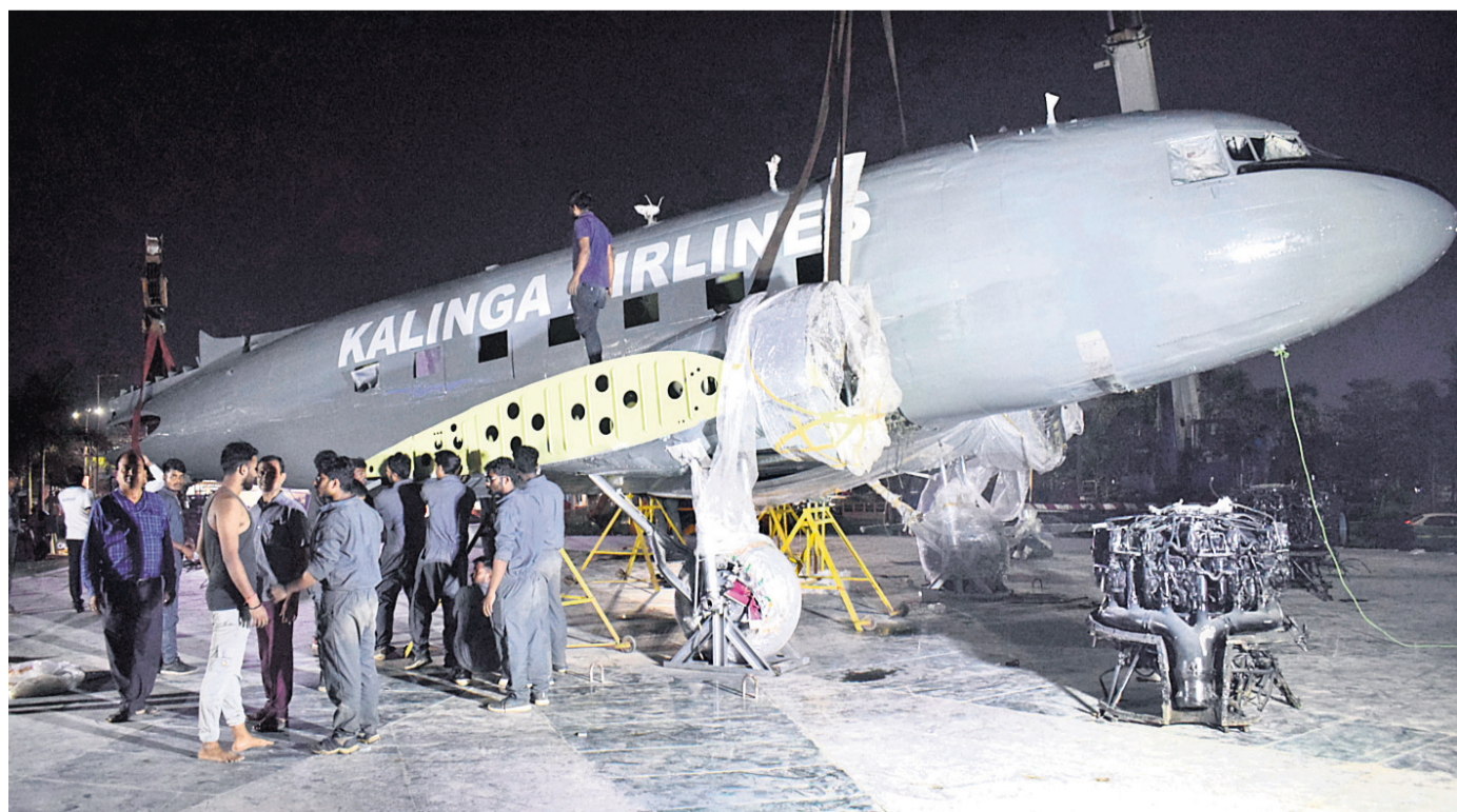
CONSERVATION BID: Former chief minister Biju Patnaik's iconic Dakota aircraft fell down while being installed through a crane at Bhubaneswar airport, Wednesday. Two persons sustained minor injuries in the incident
