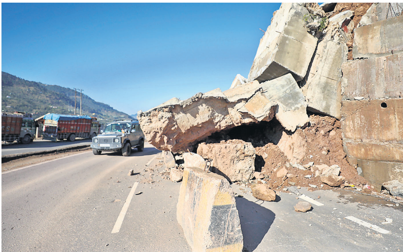
A damaged wall along the Jammu and Kashmir national highway due to landslide after heavy rainfall in Samroli area, Jammu and Kashmir
