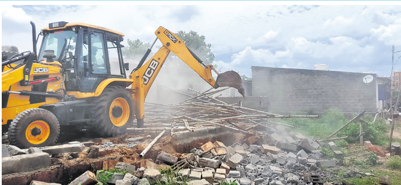
RAZING DOWN: An excavator engaged by BDA pulling down an illegally constructed house at Shyampur under Bharatpur police station in Bhubaneswar, Thursday
