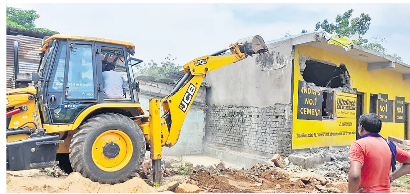
ACTION AGAINST ENCROACHMENT: An excavator deployed by BDA razing down an unauthorised structure at Jayadev Vihar in Bhubaneswar, Saturday OP PHOTO
