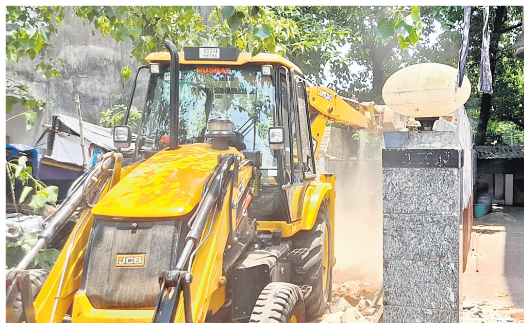
EVICTON DRIVE: An excavator deployed by BDA razing down unauthorised shops including boundary wall at Paika Nagar in Bhubaneswar, Tuesday
