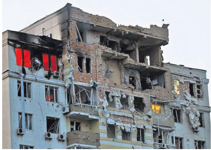
A view shows an apartment building damaged during a massive Russian drone strikes in Kyiv
