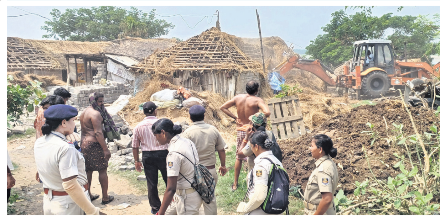
VICTION DRIVE: An excavator deployed by CMC pulling down shanties near Khannagar Kali Bhawan in Cuttack, Tuesday
