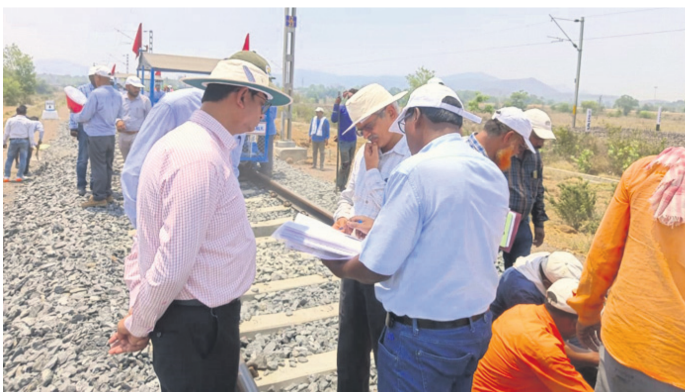
FOR PASSENGER SAFETY: Senior officials of South-Eastern Railways reviewing the ongoing expansion work of Talcher-Sambalpur rail route project between Maneswar and Sambalpur city stations. The crucial project has reached its last leg. OP PHOTO
