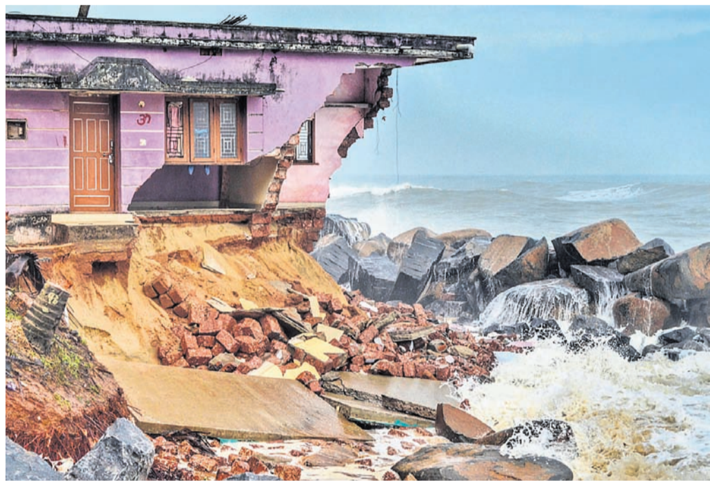
A guest house damaged due to sea erosion, at Battampady on the outskirts of Mangaluru, Sunday
