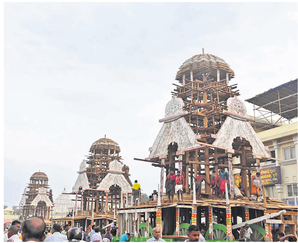
Construction of chariots of Lord Jagannath and His siblings nearing end at Rath Yard in Puri, Wednesday
