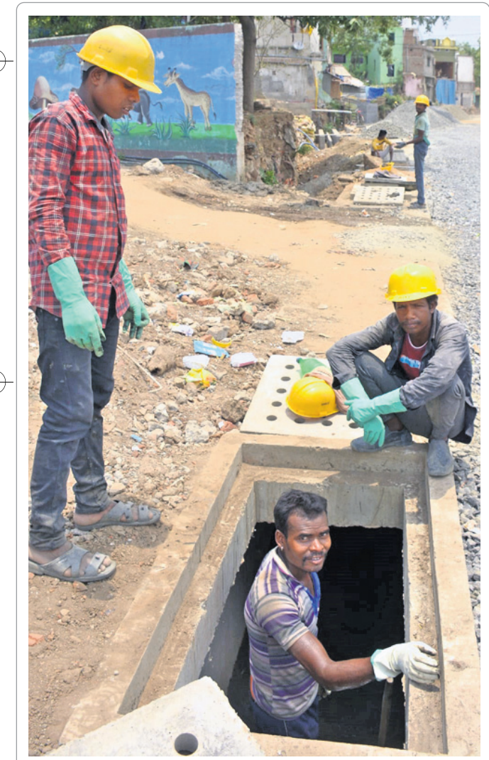
BRAVING THE SUN: Workers clean a drain in scorching heat near Samaleswari Temple in Sambalpur, Wednesday
