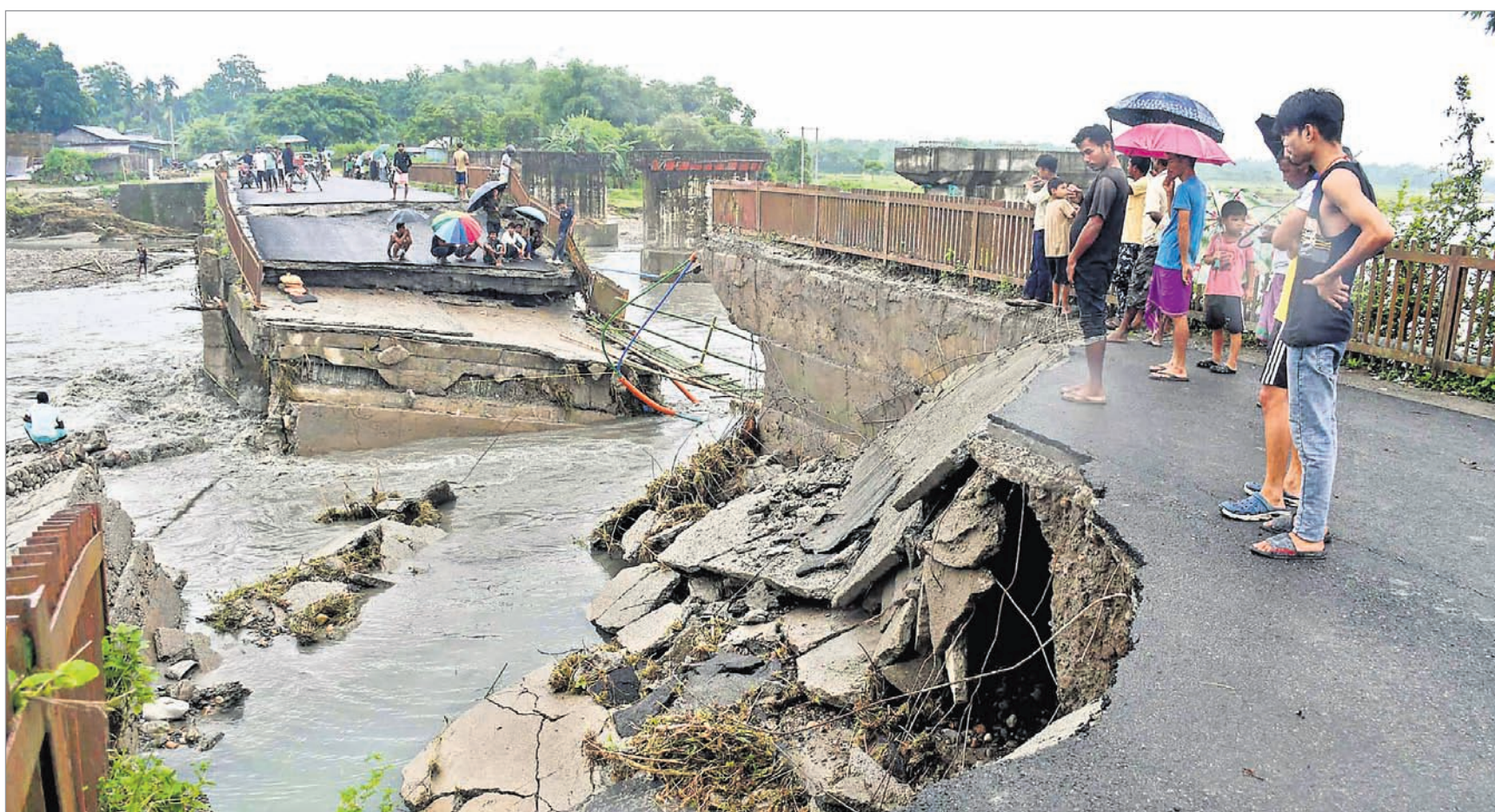
DESTROYED BY DELUGE: Villagers gather near a collapsed bridge over the Daranga River at flood-hit Kumrikata in Baksa district of Assam, Friday
