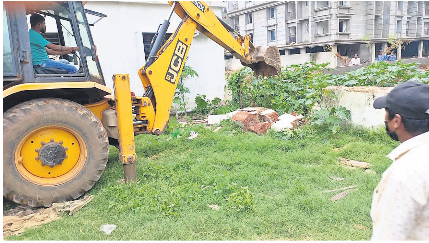
ANTI-EVICTION DRIVE: An excavator razing down unauthorised constructions including boundary wall at Jharapada in Bhubaneswar, Friday
