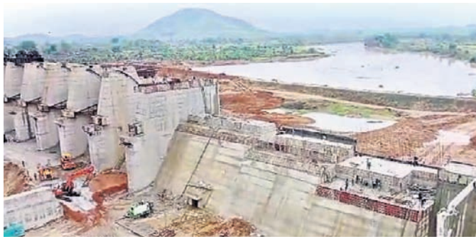
The project had to encounter many roadblocks and finally, after much uncertainty, construction of the project has reached its last leg
