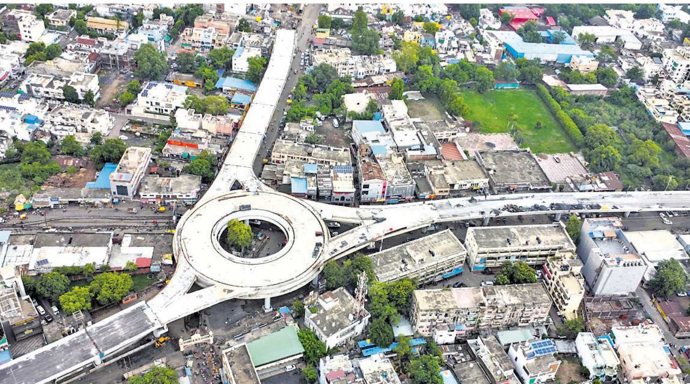
Madhya Pradesh's under-construction flyover from Damoh Naka to Madan Mahal area, that is said to be one of the longest bridges in the state with a stretch of 8 km, in Jabalpur
