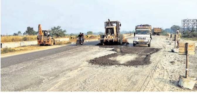
Completed by December, this year. This was stated here by project director N Nageswar Rao of National Highway Authority of India (NHAI) to this correspondent, Wednesday. Works on the bridge were first assigned to a consultancy agency Gayatri Constructions. However, the project failed to make any headway after the agency stopped
