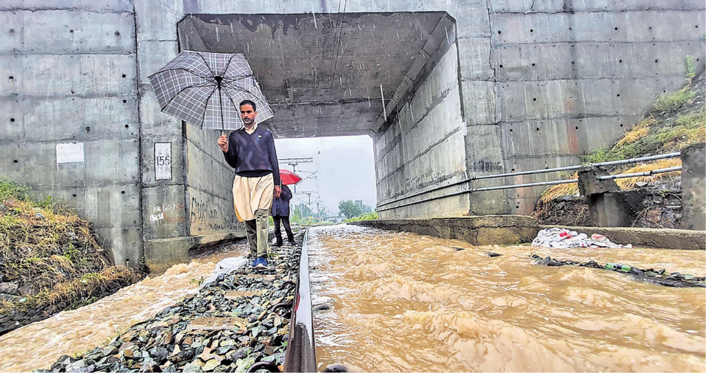
People holding umbrellas walk along railway tracks in Banihal. Rail services between Banihal and Kashmir were temporarily suspended due to rains which caused waterlogging on the tracks at several places
