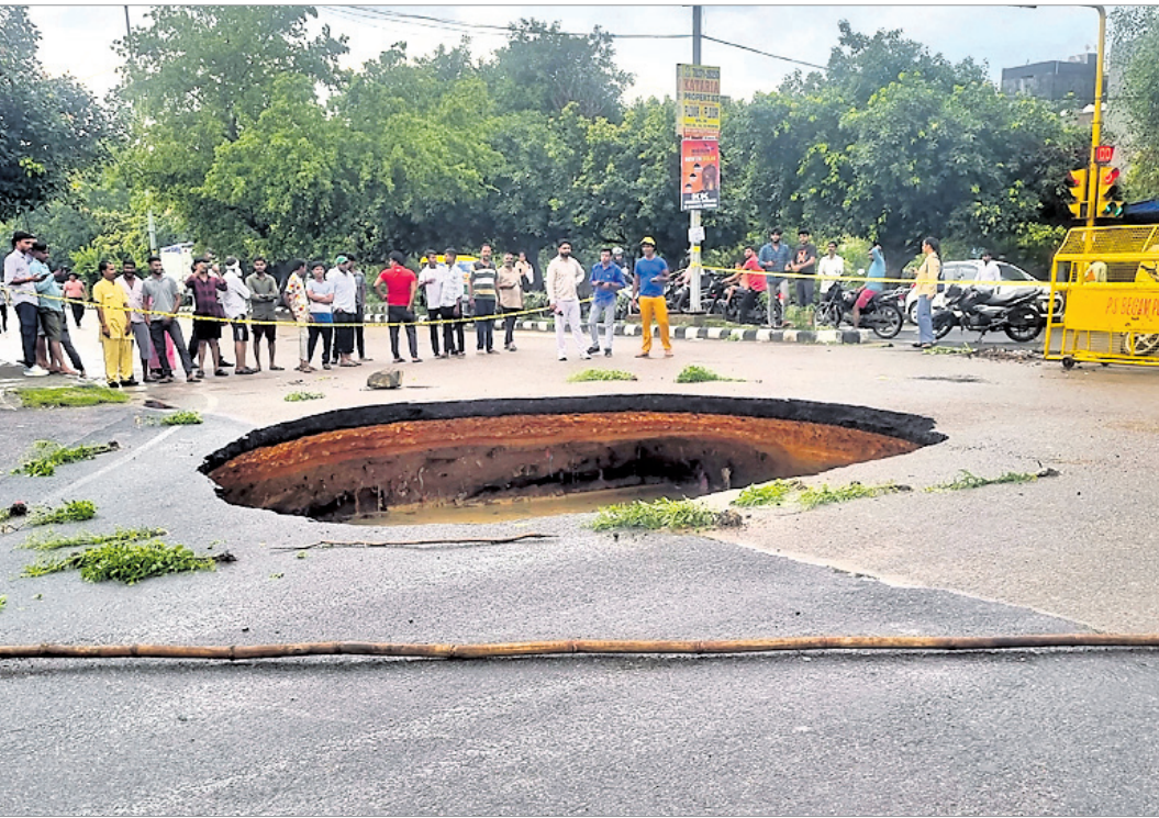
A crater is formed after a road caved in after heavy rain at Rohini in New Delhi
