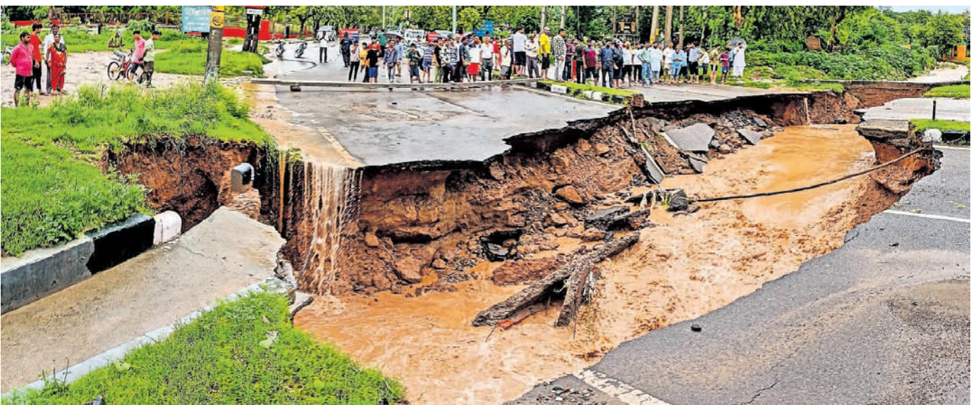
A section of a road washed away due to heavy rainfall in Panchkula, Haryana
