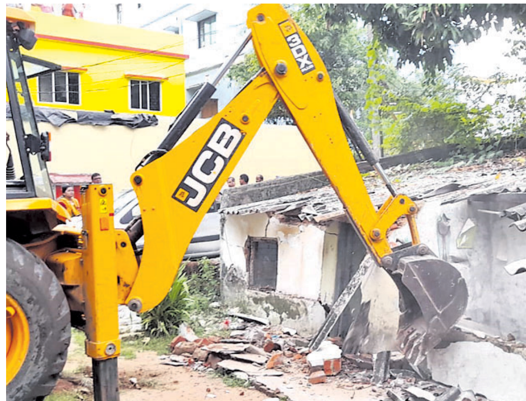
ANTI-ENCROACHMENT DRIVE: An excavator deployed by BDA razing down unauthorised constructions in Nicco Park area of Bhubaneswar, Monday OP PHOTO
