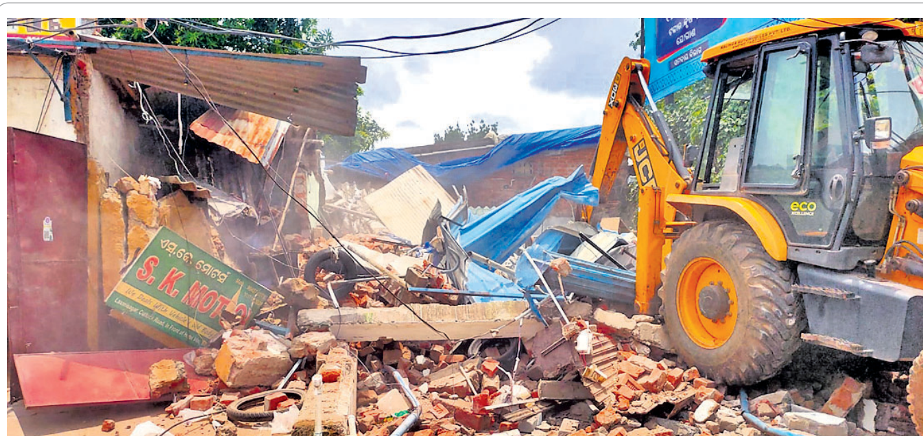
EVICTON DRIVE: An excavator engaged by BDA razing down unauthorised constructions in Cuttack Road area of Bhubaneswar, Friday
