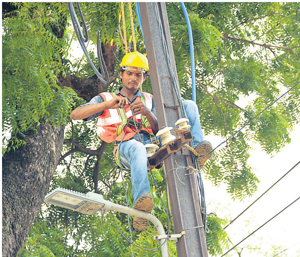
RISKY PROPOSITION: An technician working on a power line in a hazardous condition at Kacheri Square in Sambalpur, Friday
