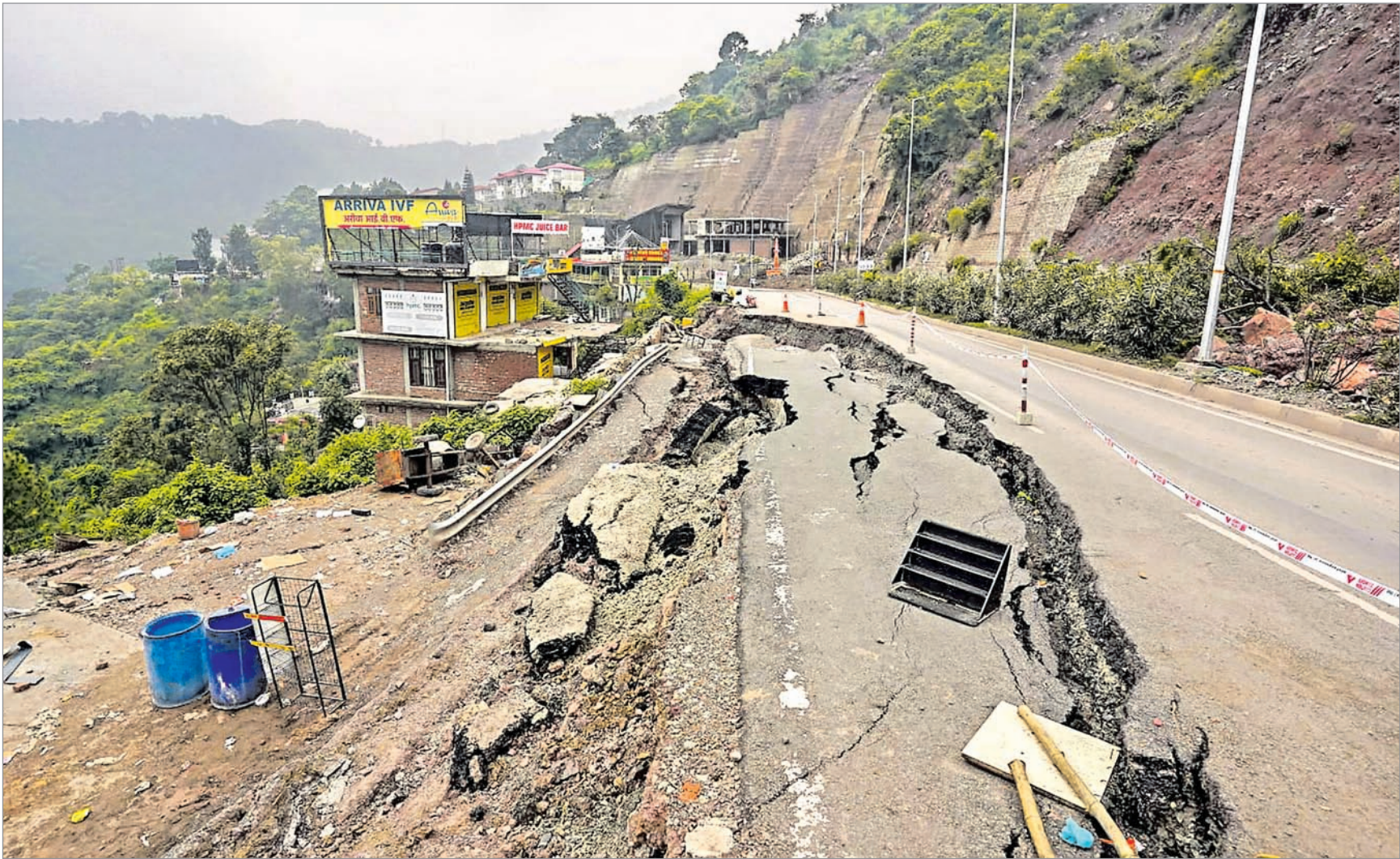
MONSOON MAYHEM: Damaged Shimla-Kalka National highway near Dharampur in Solan district of Himachal Pradesh after a flood following heavy rain, Saturday
