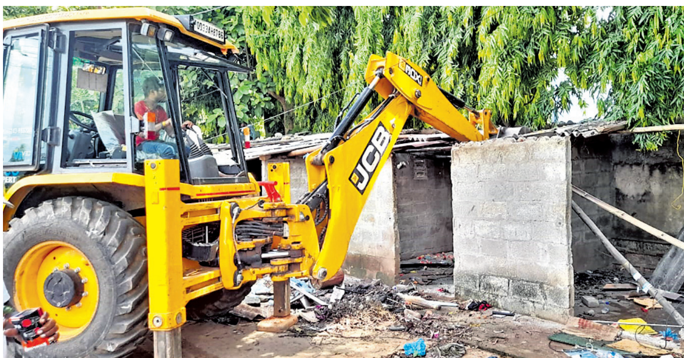
EVICION DRIVE: An excavator deployed by BDA razing down unauthorised constructions in Kalinga Studio Square area of Bhubaneswar, Tuesday
