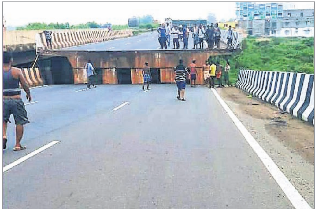
Portion of a bridge near Rasulpur block office in Jajpur district on National Highway-16 connecting Chennai and Kolkata caves in, Tuesday
