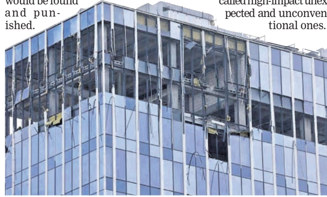
A view shows a damaged building following the reported drone attack in Moscow, Russia
