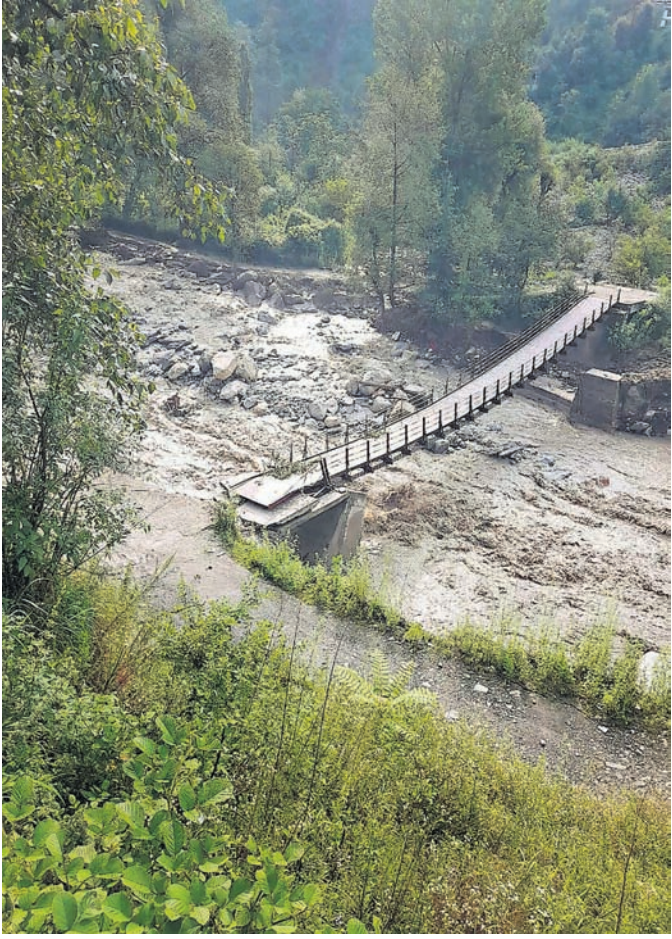
A portion of a bridge damaged due to a cloudburst during monsoon season in Gadsa valley in Kullu district, Himachal Pradesh
