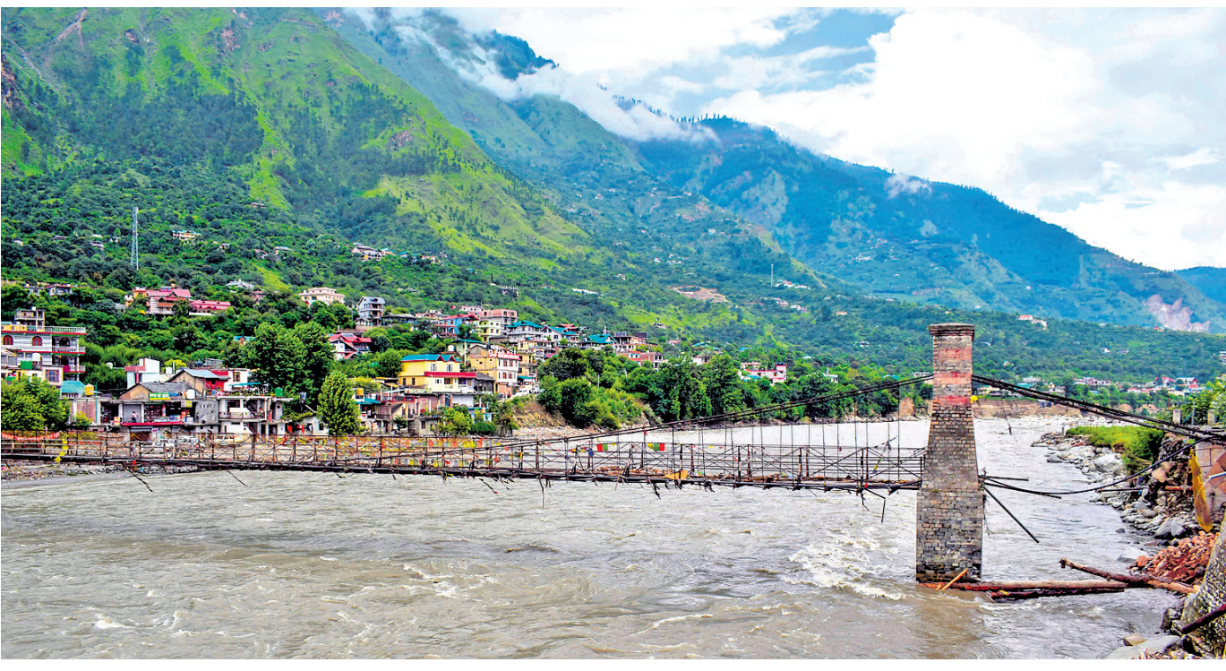
RAIN WOES: The swollen Beas River flows in spate beneath a damaged bridge at Bhuntar after heavy monsoon rains in Kullu district, Himachal Pradesh. PTI PHOTO
