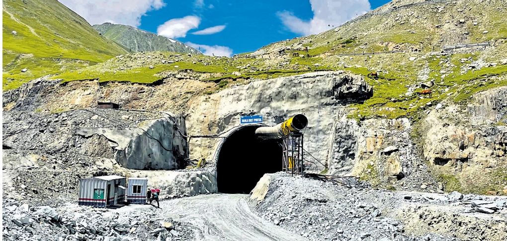
Construction work underway at Asia's longest bi-directional Zojila Tunnel at Baltal area in Ganderbal district
