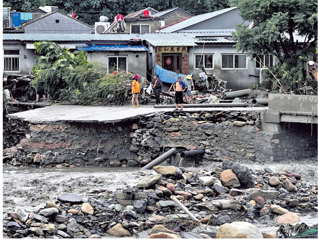
Villagers look at a collapsed road damaged by floodwaters in the Mentougou district as continuous rainfall triggers alerts in Beijing
