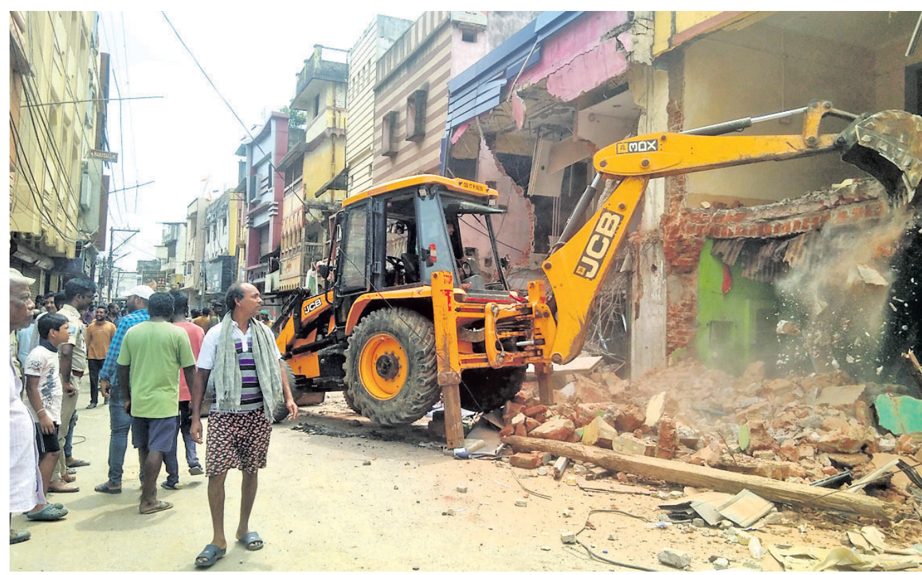
EVICTON DRIVE: An earthmover demolishing an illegal construction to clear encroachments from Lengu Mishra Square till New Jeera bridge road in Bargarh, Monday
