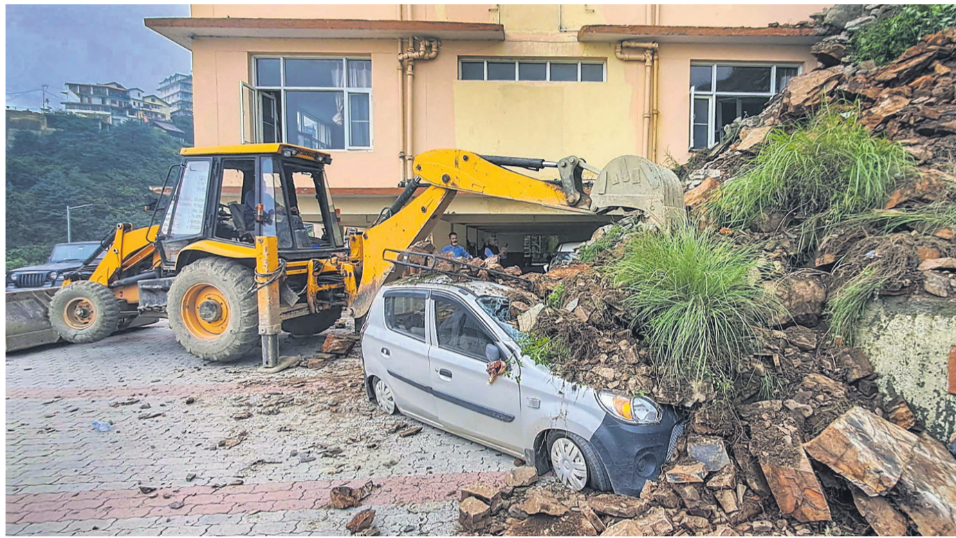
A backhoe machine removes the debris that fell upon a vehicle due to a landslide triggered by heavy monsoon rains in Shimla, Himachal Pradesh PTI PHOTO
