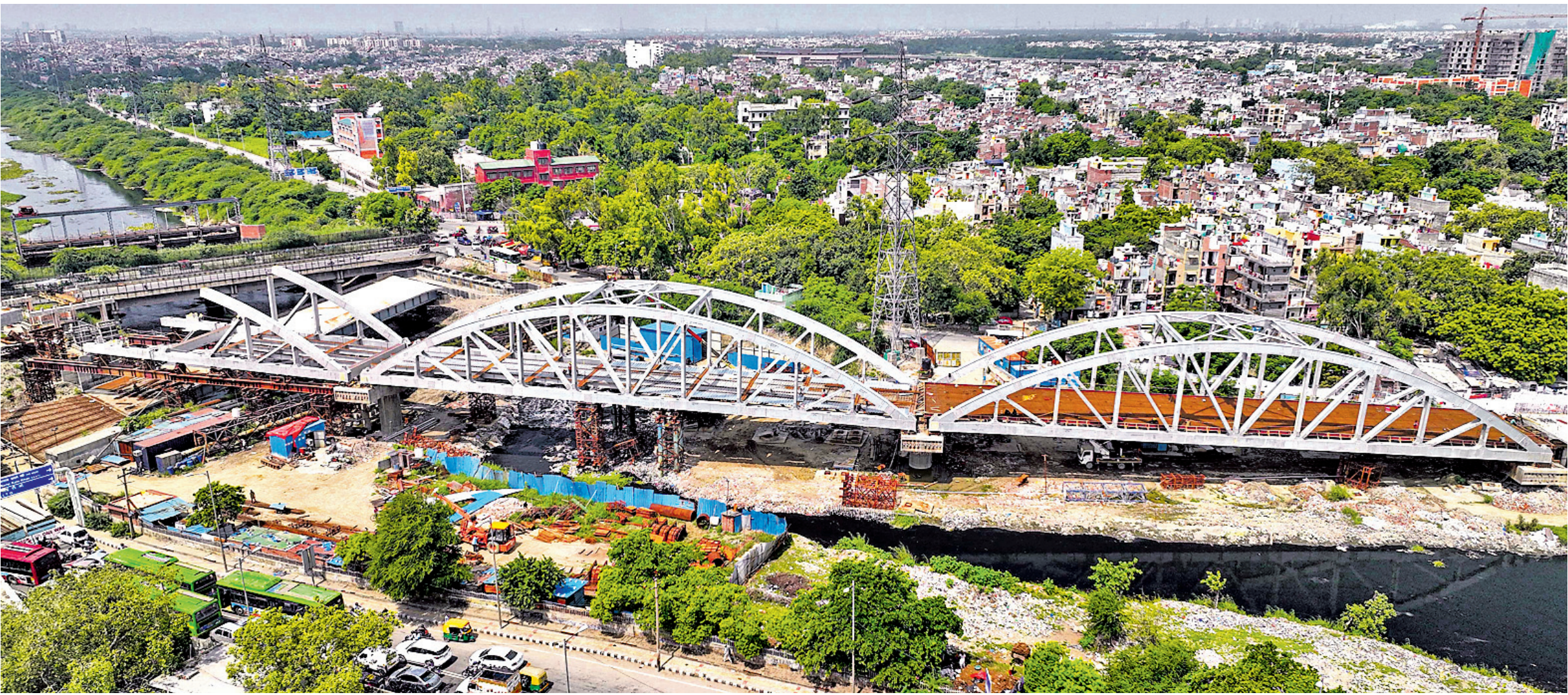
Special steel spans installed on the Regional Rapid Transit System (RRTS) corridor, at Kondli in New Delhi. The steel spans are being installed where the corridor will cross Ghazipur drain from Ashok Nagar towards Anand Vihar
