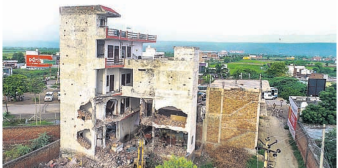
Authorities demolish the Sahara Family restaurant from where stones were allegedly pelted on a religious procession on July 31 which led to violence in Nuh
