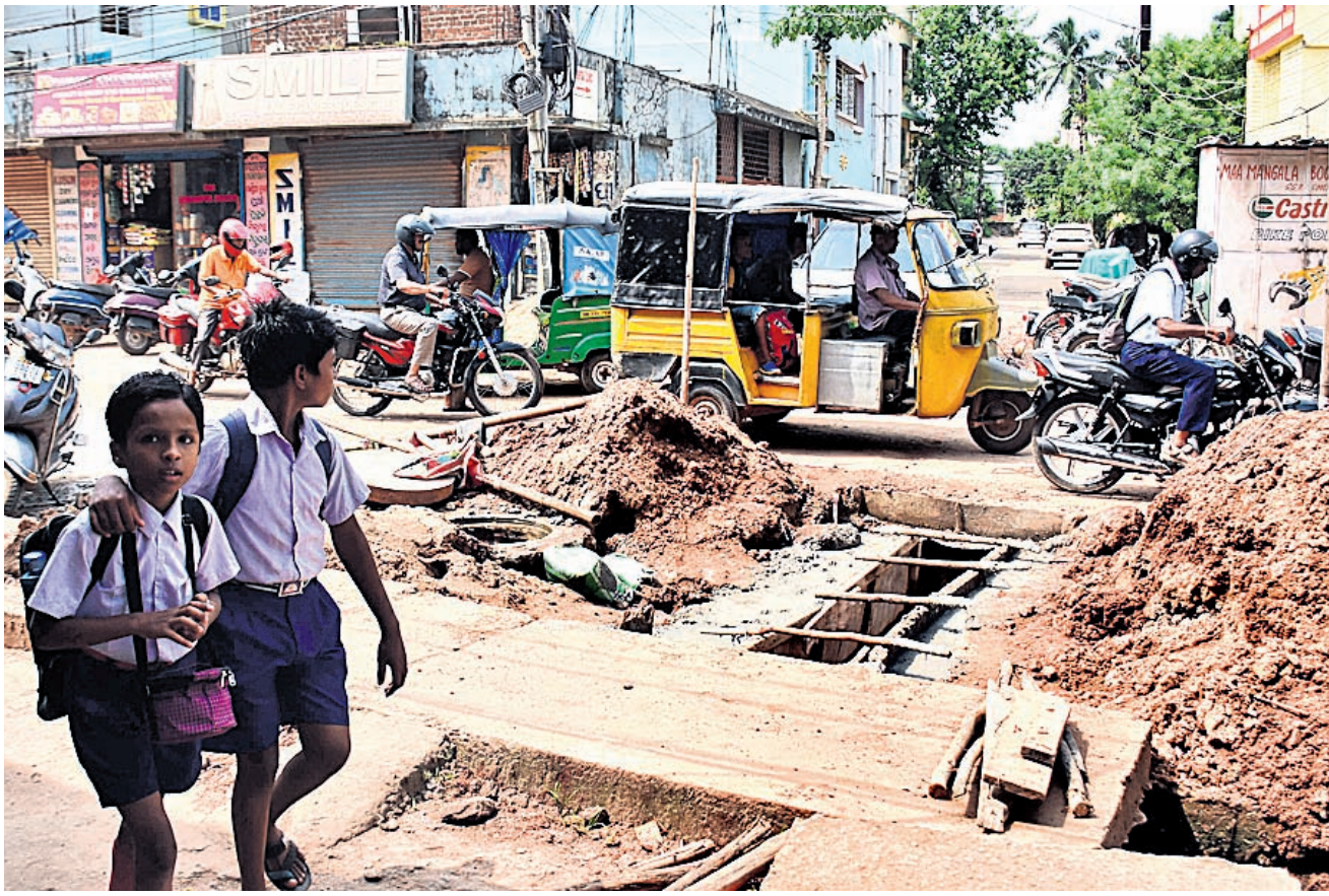
IGNORING SAFETY: A stretch at GGP Colony near Rasulgarh in Bhubaneswar was dug up for construction of drains. The site without any barricades poses threat to commuters including children
