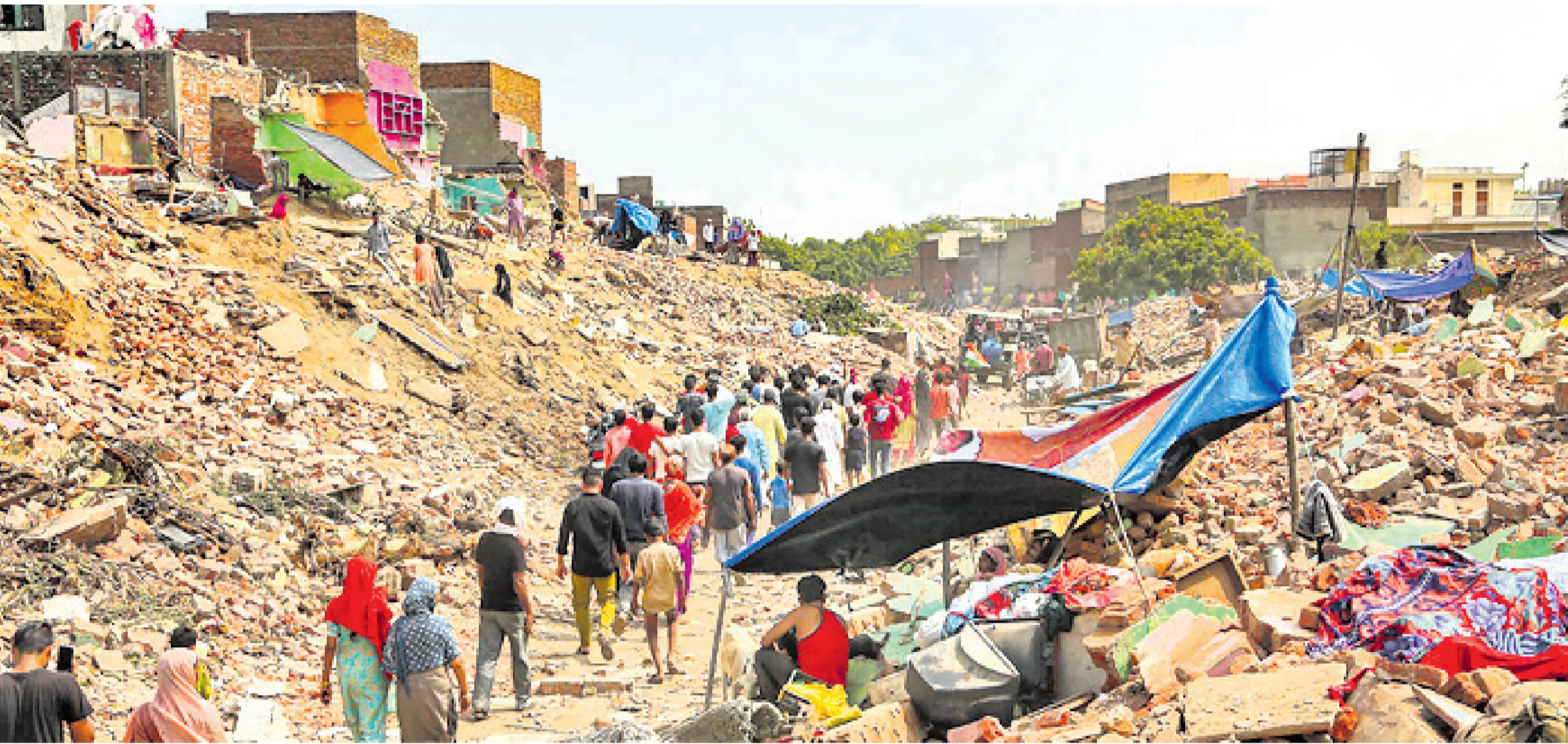
The razed houses near Sri Krishna Janmabhoomi in Mathura. The Supreme Court Wednesday ordered status quo with regard to the demolition drive being carried out by railway authorities to clear alleged illegal constructions
