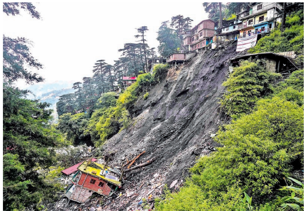
A landslide affected area where several buildings were damaged after heavy rains, at Krishna Nagar ward in Shimla
