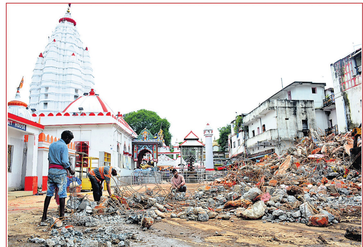
AT FULL THROTTLE: Labourers clearing the debris after the residence of the chief priest was demolished to make way for infrastructure under the SAMALEI (Samaleswari Temple Area Management and Local Economic Initiative) project on Samaleswari temple premises in Sambalpur, Friday
