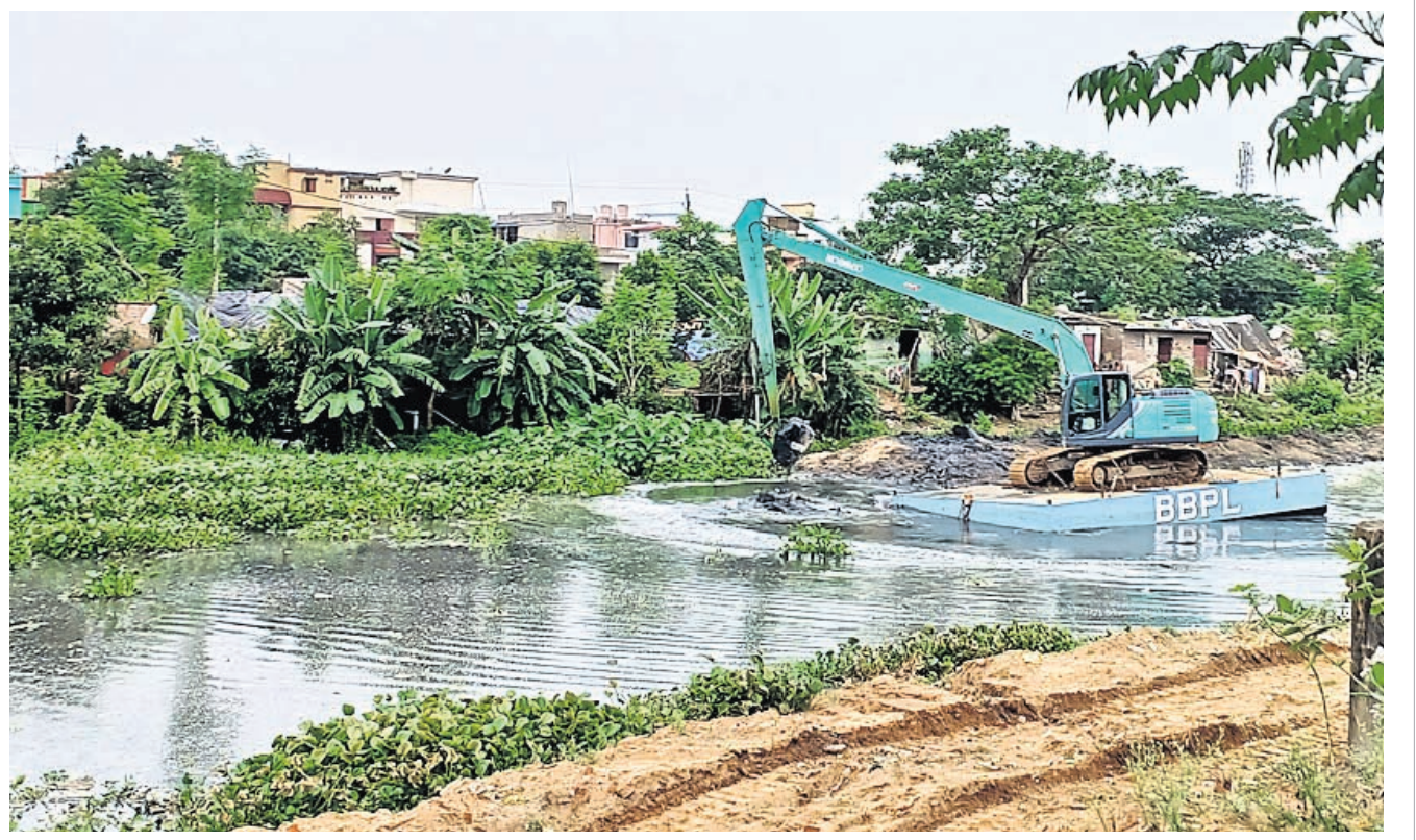
CANAL REJUVENATION: An excavator engaged by CMC removes weeds from Petanala in CDA area of Cuttack, Friday
