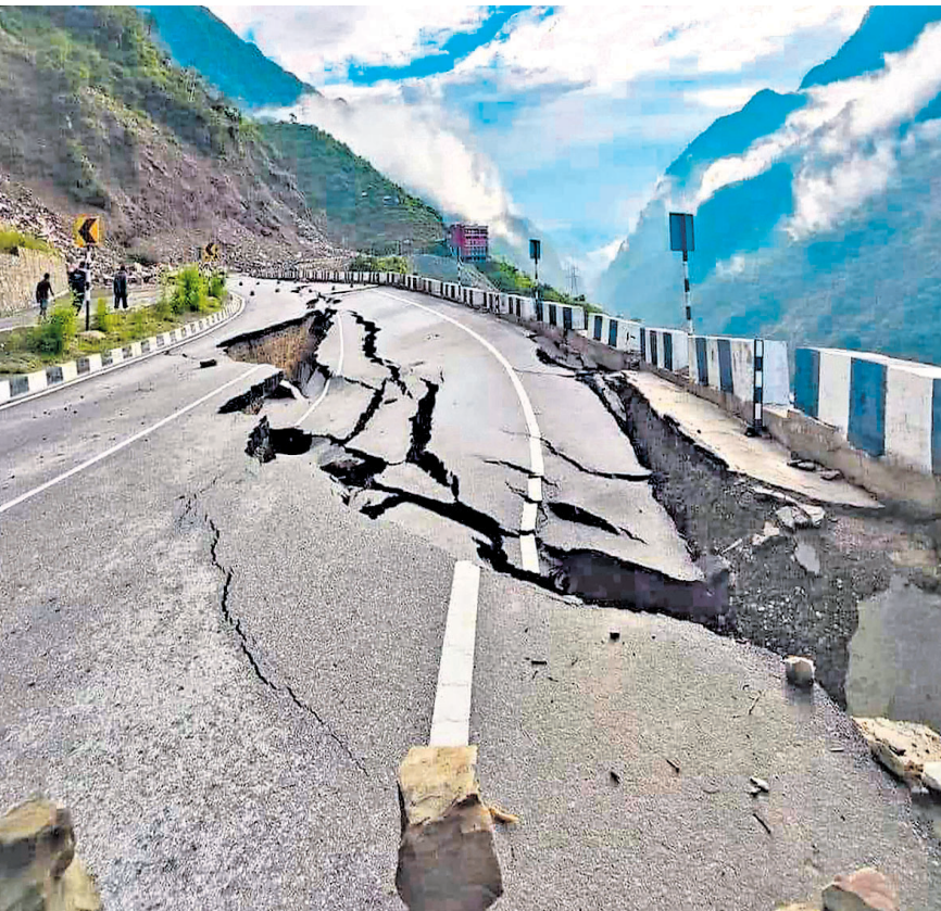
Damaged Kiratpur-Manali road following heavy rainfall, near Pandoh in Mandi district
