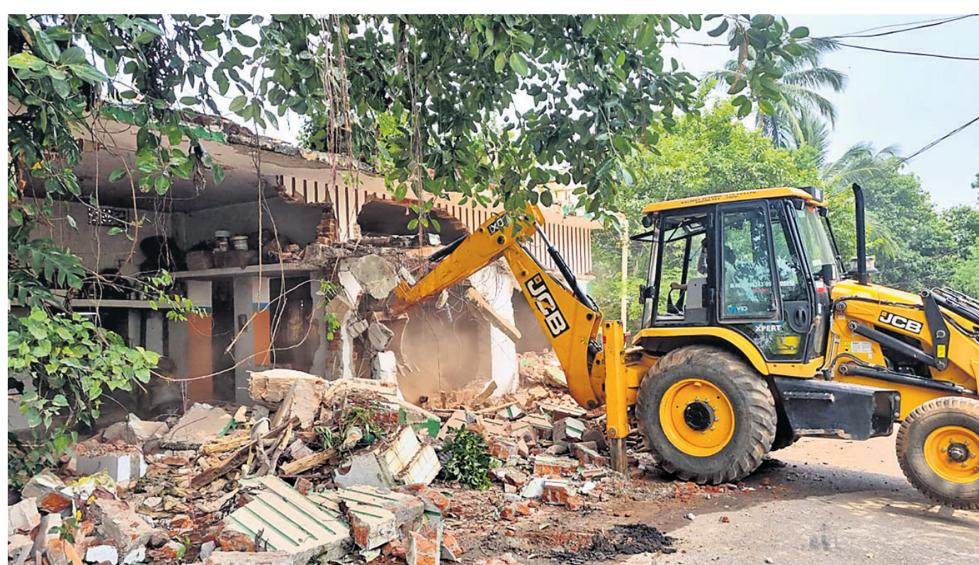
EVICTON DRIVE: An excavator deployed by BDA razing down an illegal construction at Kharavela Nagar in Bhubaneswar, Tuesday
