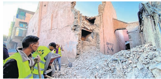
People work next to damage in the historic city of Marrakech, following a powerful earthquake in Morocco REUTERS
