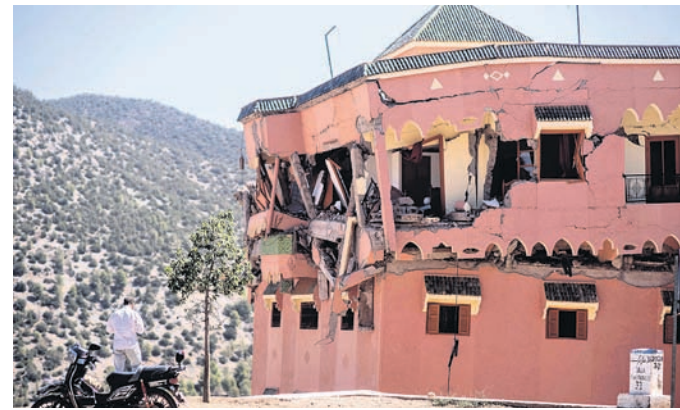
A man stands next to a damaged hotel after the earthquake in Moulay Ibrahim village, near the epicentre of the earthquake, outside Marrakech PTI PHOTO
