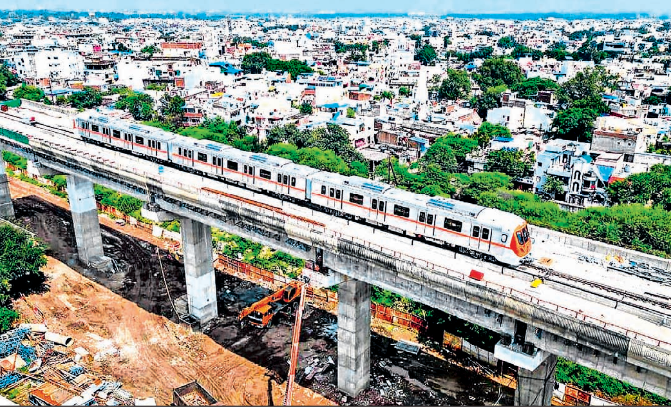
A metro train being put on the track for a trial run from Subhash Nagar Depot to Rani Kamalapati Railway station in Bhopal, Madhya Pradesh
