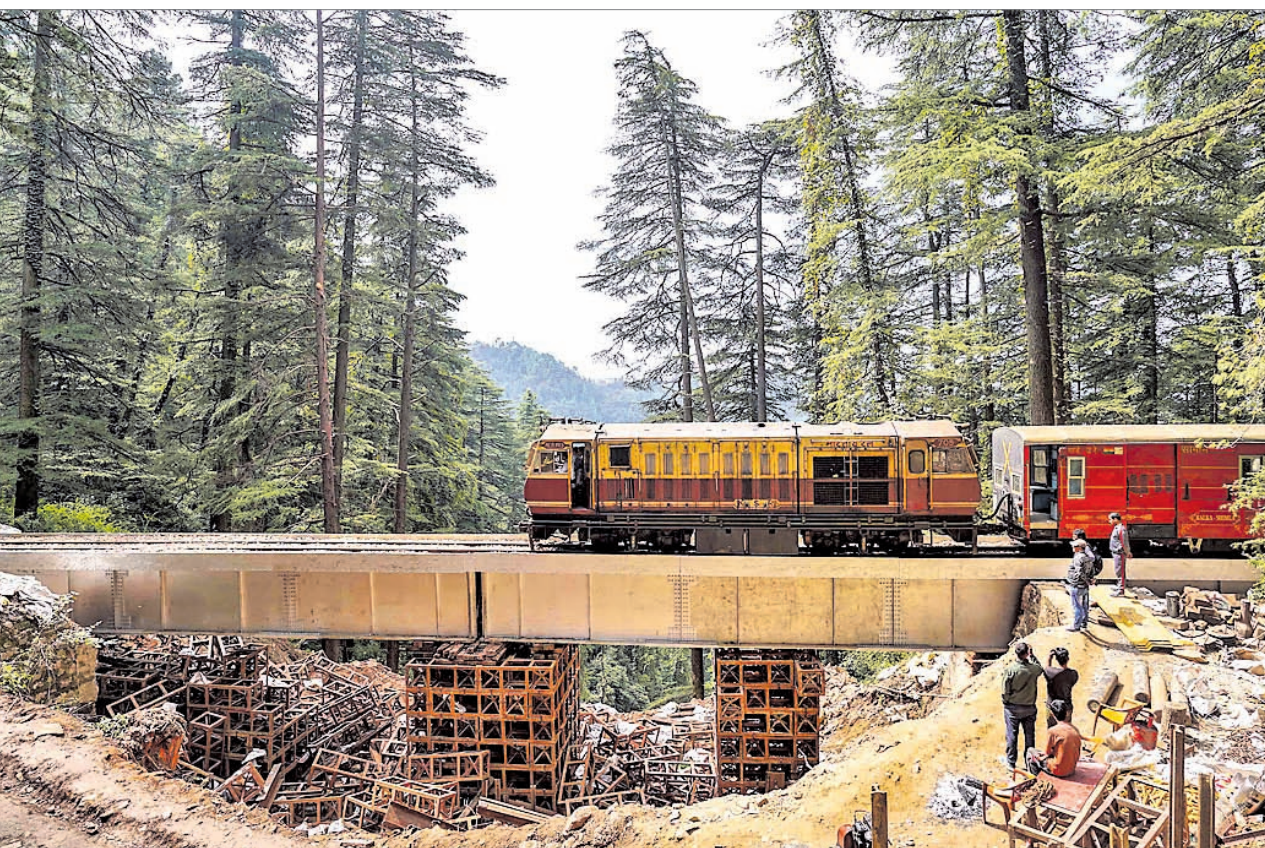
A toy train runs on the Kalka Shimla Heritage Rail track after installation of plate girder bridge near Summerhill railway station where bridge and rail track was totally damaged due to landslides August 14
